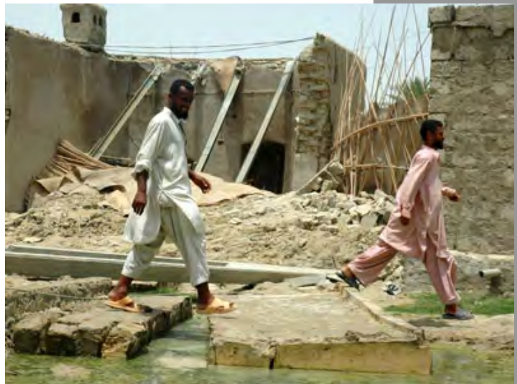
Two men walk along a broken concrete sanitation drain in Nokalat, Pakistan. Photo: Mubashir Fida/ International Federation
